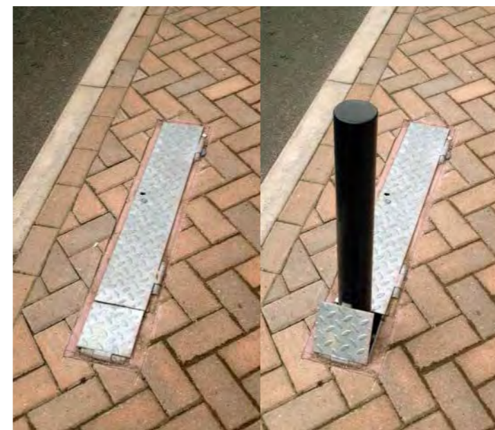
Figure 33: Drop-bollard vehicle access barrier.
