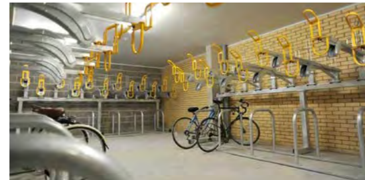
Figure 20: Hydraulic stacking cycle racks within secure internal areas.
